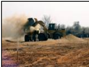
Medupi coal fired power station in Lephale
