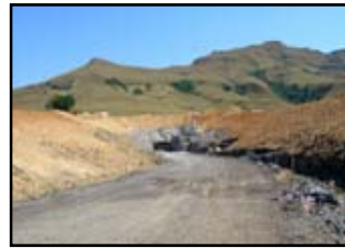
Ingula pumped storage scheme near Ladysmith
